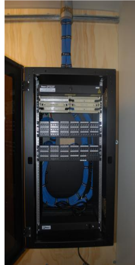
Enclosed and lockable cabinet mounted high on wall
